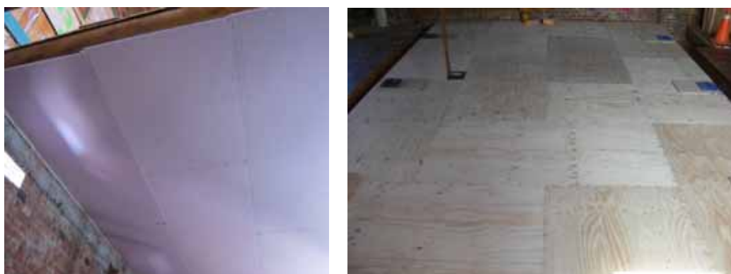
Fig. 2: a) Diaphragm retrofitted with a plywood panel overlay; b) fire rated ceiling lining
