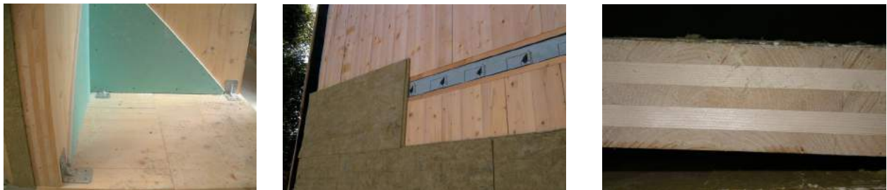
Fig. 76 Additional lining, OSB Strip at the end face or the use of tight panels
