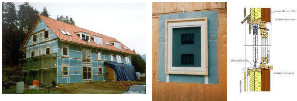
Fig. 57 Example for an airtightness solution with a convection inhibiting foil beyond the exterior thermal insulation. (not necessary for tight CLT panels)
