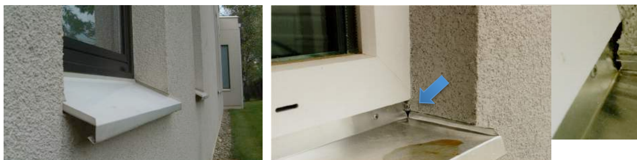
Fig. 32 Left fig.: Splash-proofed window sill; right fig.: Bad example with a hole in the corner
