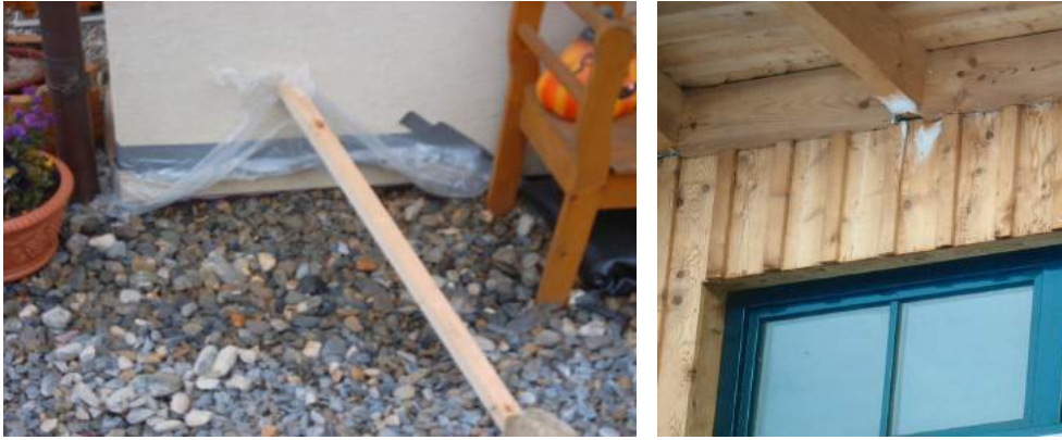
Fig. 54 Two examples for convection of dampness: Left Figure: Base gap; Right figure: Ice around a cantilever beam
