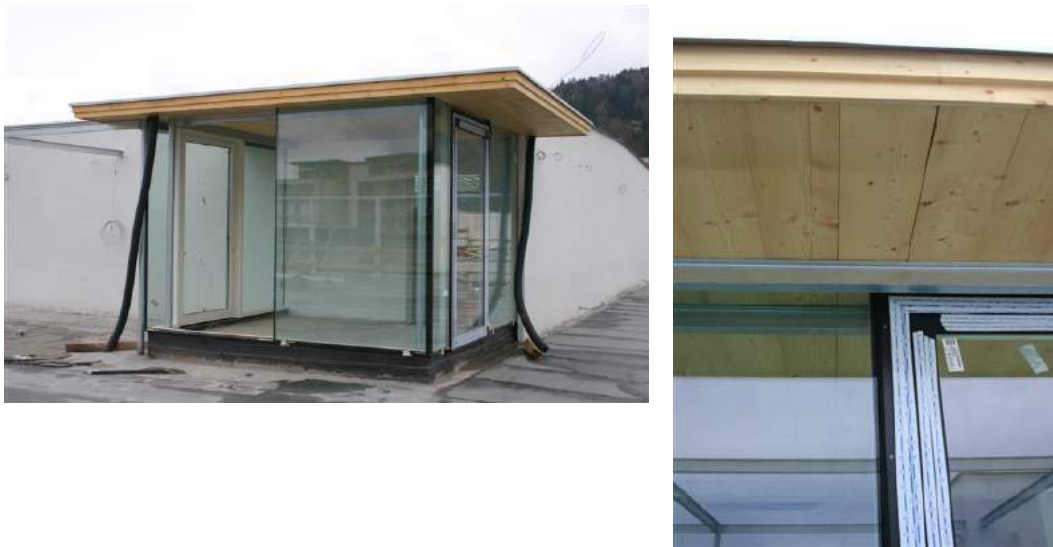
Fig. 55 Bad example of a canopy with a gap from inside to outside
