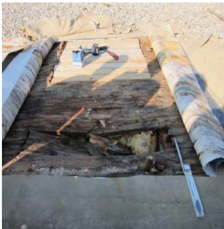
Fig. 46 Fungal damage caused by moisture in a flat roof
