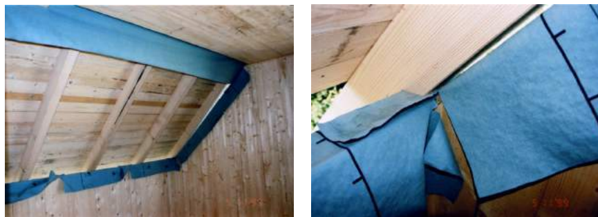
Fig. 59 Difficult airtight joint between the airtight layer and the vapour barrier of the sloping ceiling
