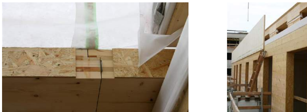
Fig. 60 Left fig.: Examples for good construction design of an exterior slab joint. The joint is covered here with an OSB-strip. Right fig.: Closing of the gap between wall and slab with a compressed sealing strip, an airtight foil and a thin three-layer panel
