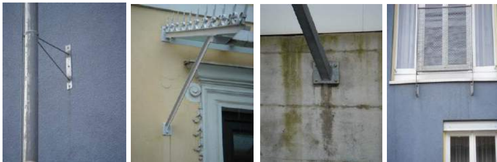
Fig. 36 Badly designed fastenings
