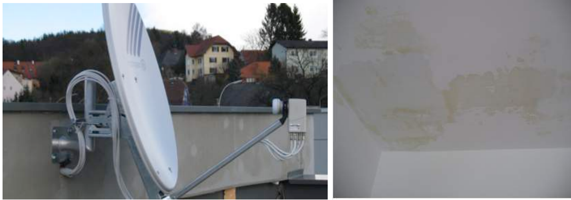
Fig. 38 Building damage caused by wrong mounting of a satellite dish and satellite dish cable
