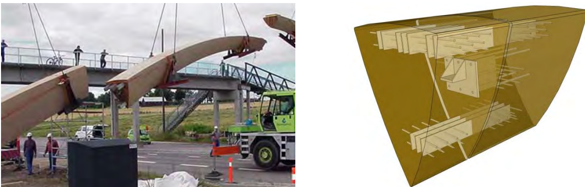
Figure 2: Leonardo Footbridge (2001), Norway, left: the central arch under assembling, right: 3D model of the splice joint
