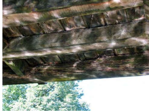
Figure 15: Deteriorated main beam
