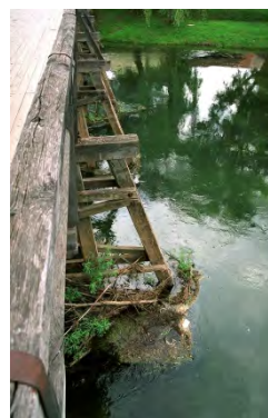
Figure 9: Deteriorated railing and river debris
