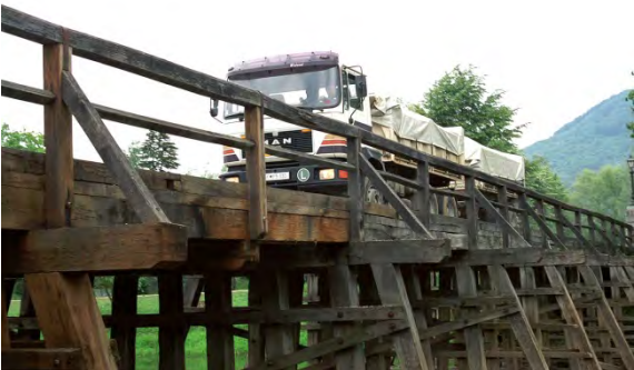
Figure 6: Trucks overloading the bridge.
