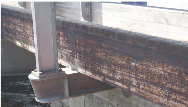
Figure 16: Structural detail which should be evaluated with respect to accumulation of dirt
