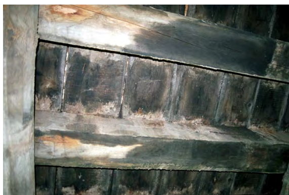
Figure 12: Fungi attack - main beams, lower deck
