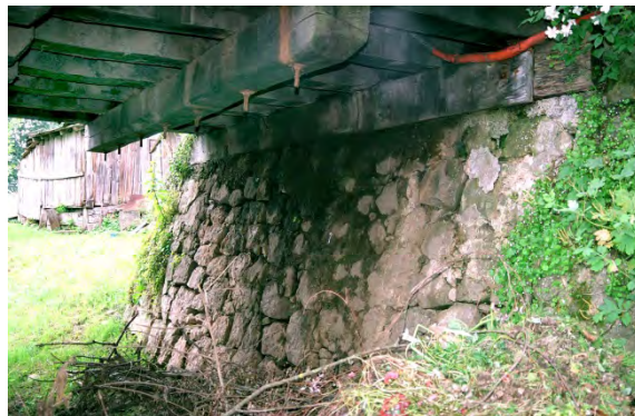
Figure 7: Corrosion of steel and cracks in stone pillar
