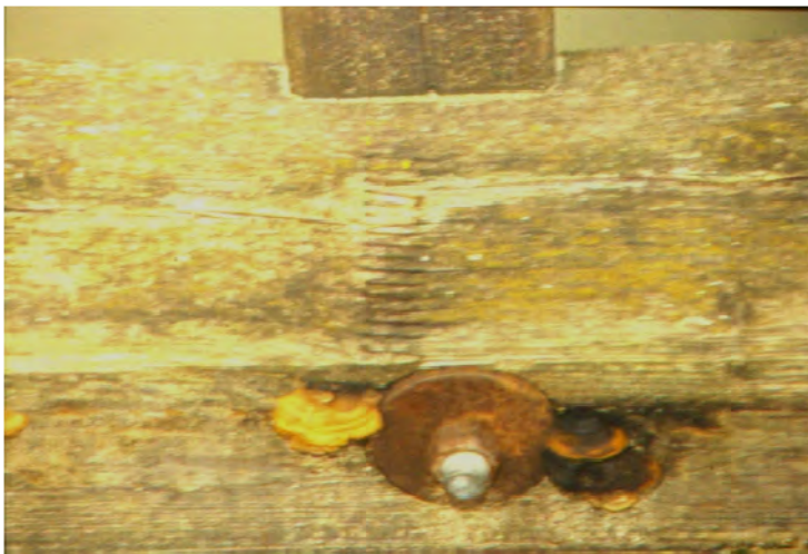
Figure 1: Timber-bridge n. 9. Fruiting bodies of brown-rot fungi, close to moisture trap (hole, bolt and washer).
