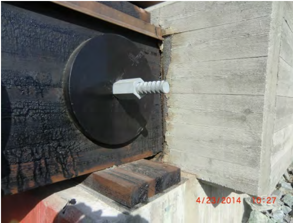
Figure 6: Structural detail which should be evaluated with respect to water trapping
