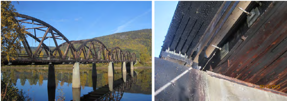
Figure 1: Left: View of Evenstad bridge. Right: detail of the stress laminated deck.
