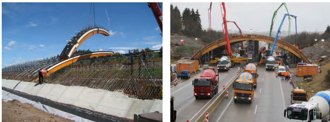
Figure 6: Building progress: adjustment of the timber ribs (left side) and concreting (right side) (photos: K.-H. Lorbach)
