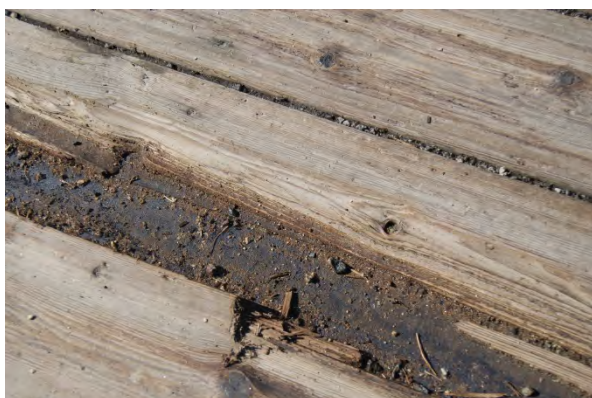
Figure 13: Damage on deck due to standing water (Måna bridge)
