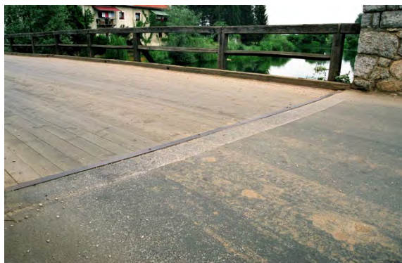
Figure 10: Dilatation profile needs retightening
