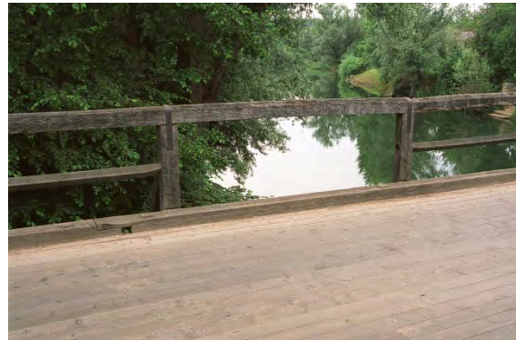
Figure 11: Part of railing is missing
