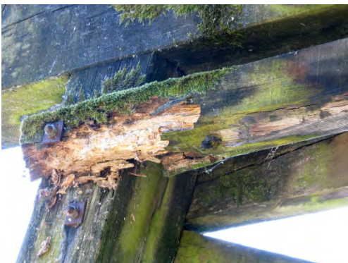
Figure 18: Deteriorated tie beam
