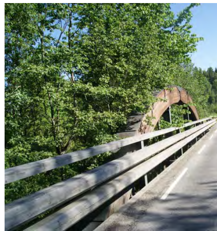
Figure 17: Vegetation touching the timber elements
