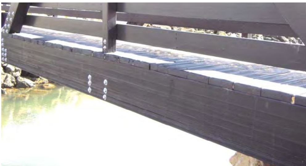
Figure 2: Crack of the timber member
