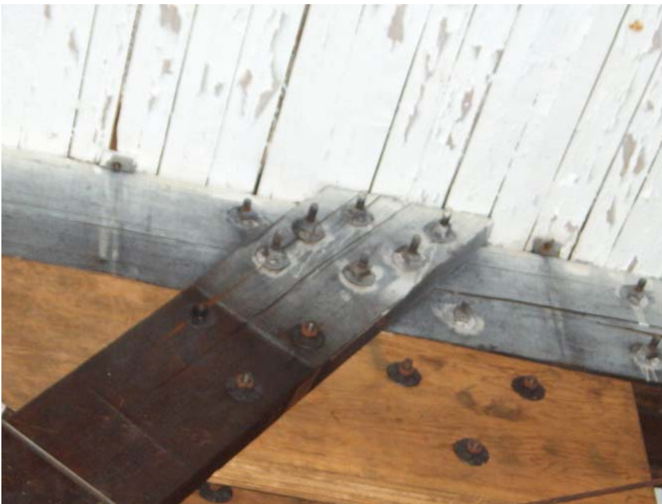
Figure 2. Shrinkage split resulting in significant reduction of connection resistance
