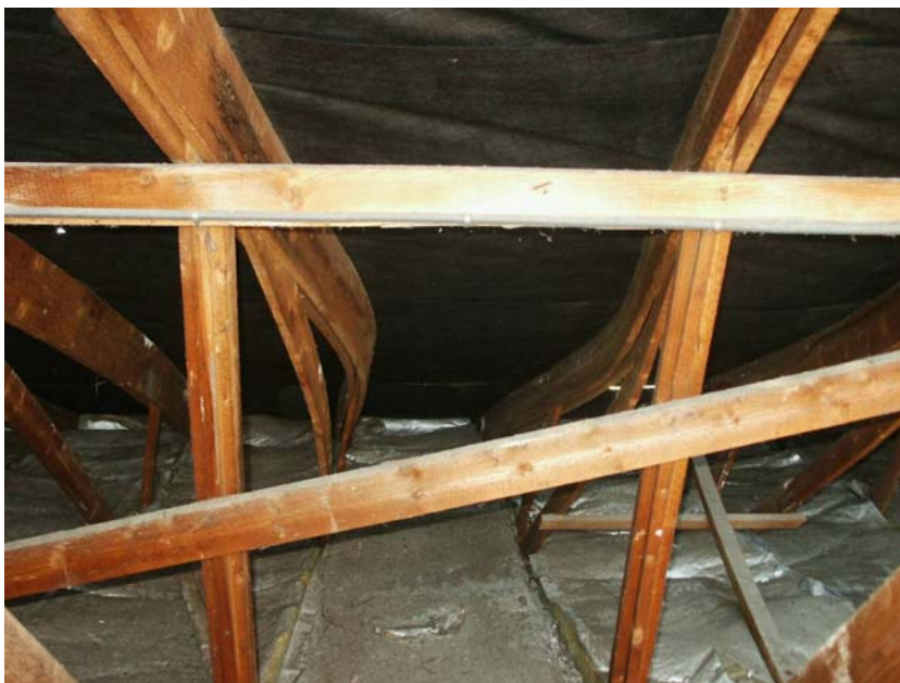
Figure 6: Buckling of compression-loaded members of a trussed girder
