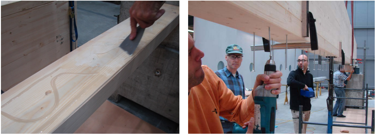
Figure 5: Screw-press bonding for the application of additional lamellae for a glulam beam. Left hand side: application of the PUR adhesive, right hand side: setting of the screws in a predefined pattern.
