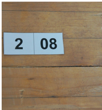
Figure 2: Delamination in the glued joint
