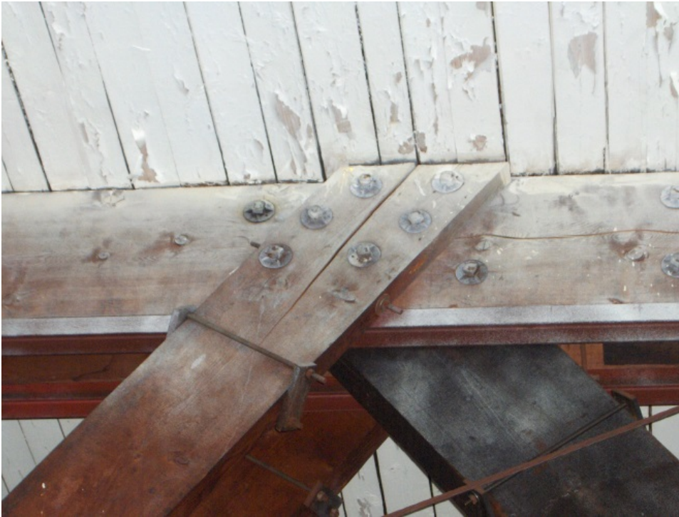
Figure 1. Shrinkage split with no effect on connection resistance
